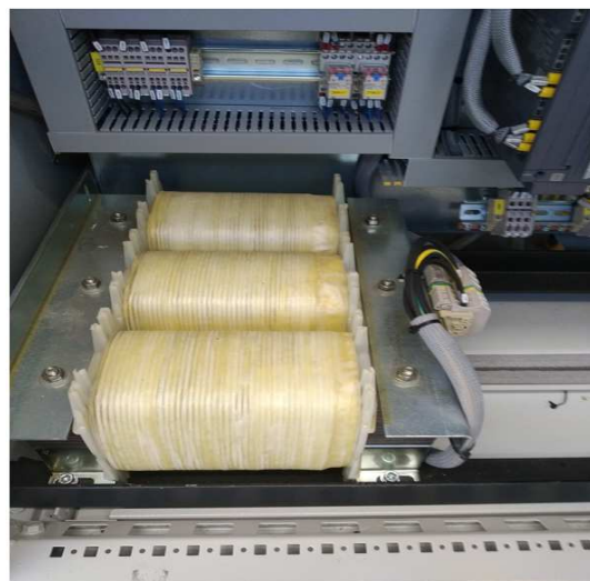
Figure 8: Transformer 400 V /210 V.
