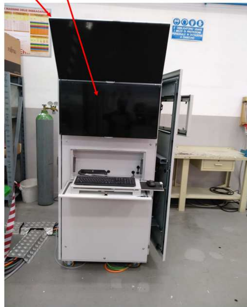
Figure 10: Controller Cabinet with Monitoring System.
