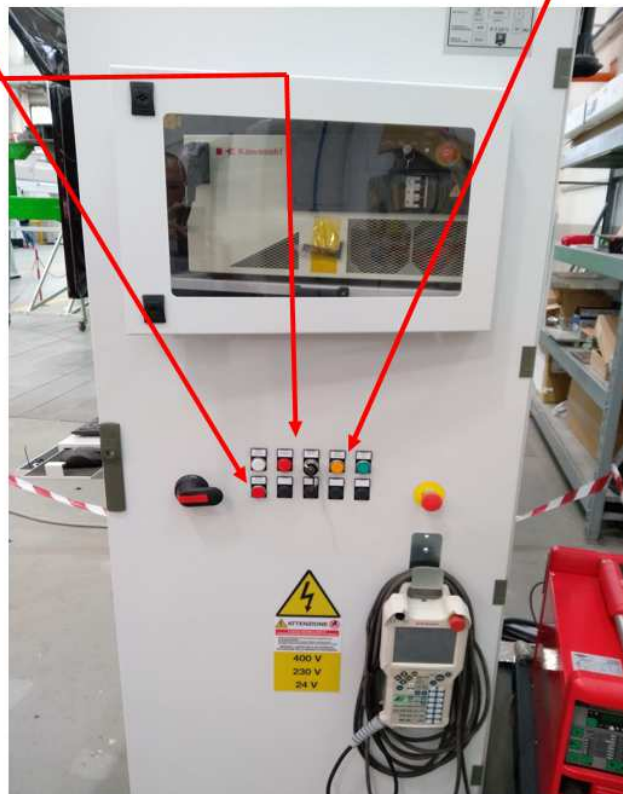
Figure 5: Lamp and Button Front Cabinet.
